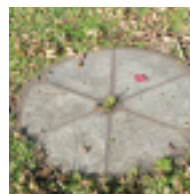
Sewer Maintenance Hole
