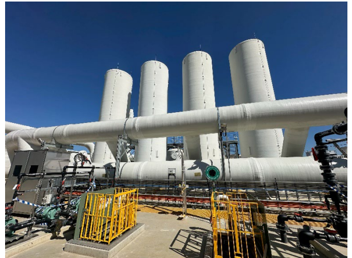
Photo 2: Odour control facility
