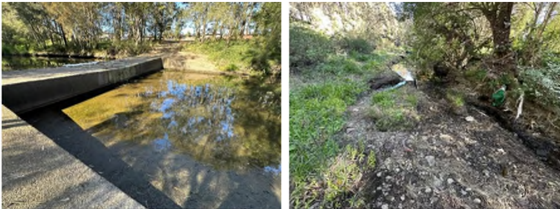
Un-culverted crossing, buildup of sediment and rubbish blocking fish passage
