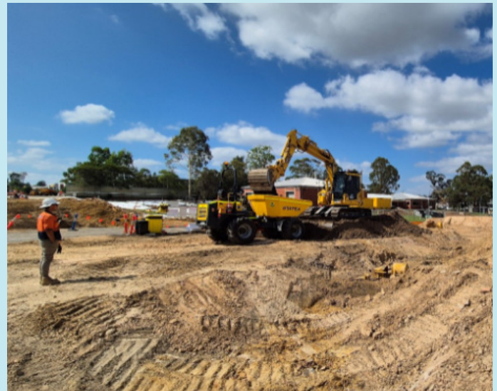
Most of the North West Treatment Hub program work will take place on site at the Rouse Hill Water Resource Recovery Facility. Pictured here is excavation work for the growth program.
