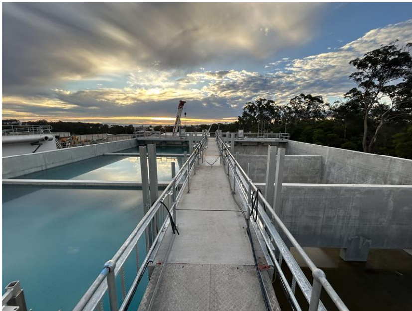
Figure 4 Anoxic tanks north empty after hydrostatic test water has been transferred to anoxic tanks south
