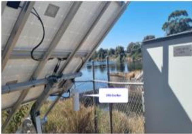
Mill Stream Outlet is located at the ERS Structure
