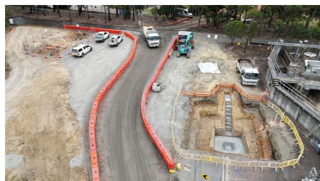
Encased brine pressure main, an important pipe within the network that pushes brine water through the plant
