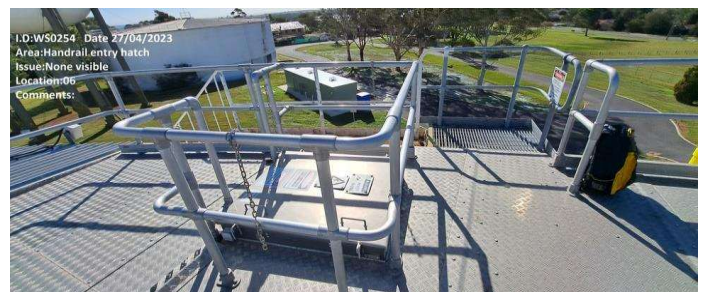
Personnel access hatch with walkway
