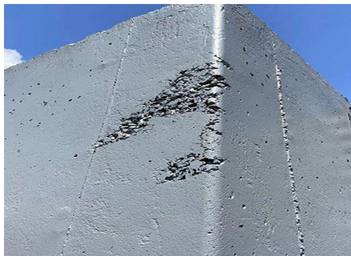
Honeycombing in concrete wall
