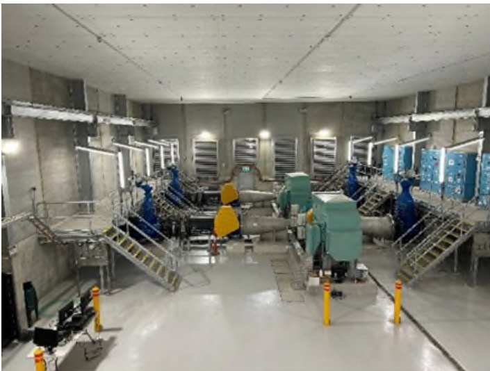
High Voltage Pump Station and Switchgear
