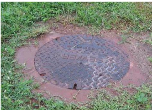
A typical maintenance hole on a private property.
