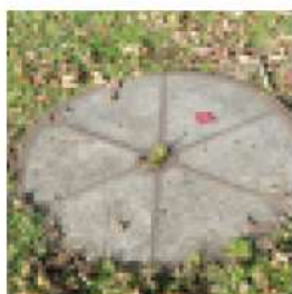
Sewer Maintenance Hole
