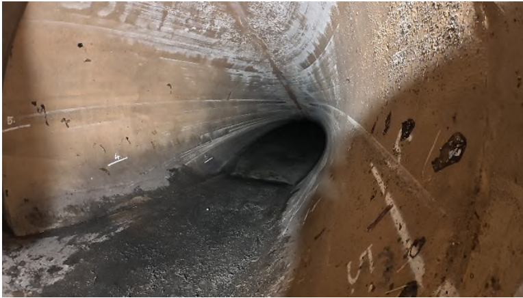
Figure 49: The decline tunnel to the North Head DOOF on the inside of the bulkhead door once cleaning had been completed
