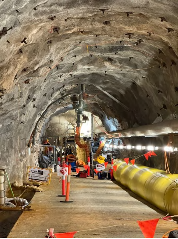
Figure 47: Example of the difficult access conditions for entering the DOOF bulkhead door
