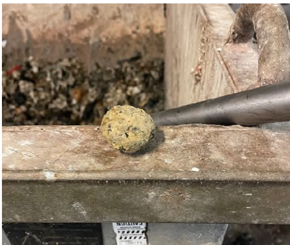
Figure 20: Example of one of several debris ball formed in the network and removed on the plant screens.
