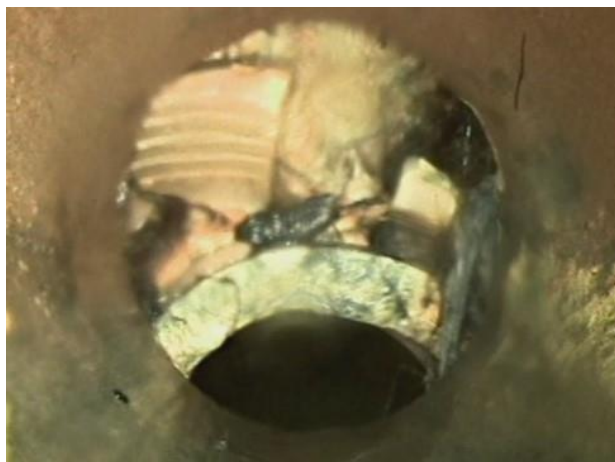
Example of clear photo evidence showing displaced and collapsed pipework at the end of a section of pipe.
