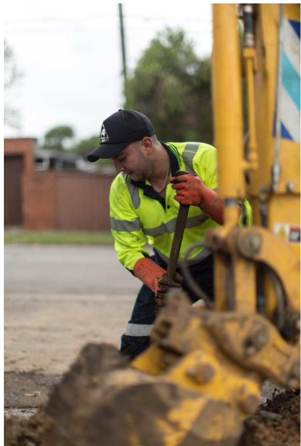
Our team can safely excavate and repair your collapsed pipes under public roadways and footpaths.
