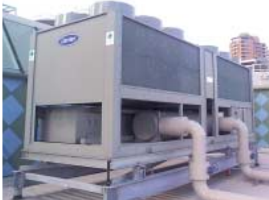
Air cooled chiller
