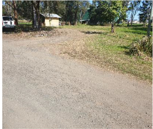
Figure 9: Unsealed residential driveway in west of study area
