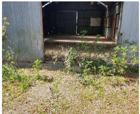
Figure 13: Agricultural shed at back of 235 South Street, showing impacts from a concrete foundation
