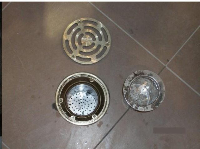
In-floor bucket trap
