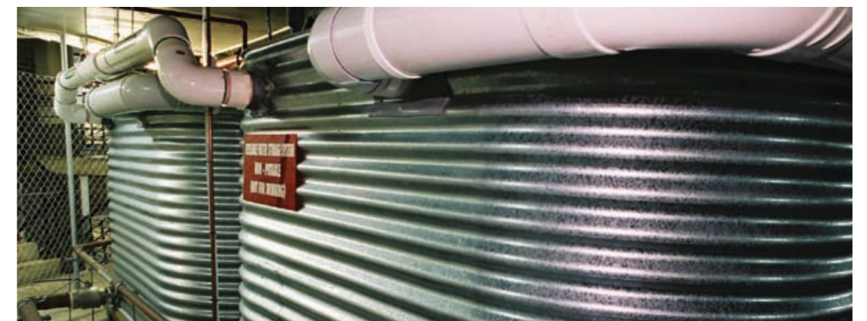
Photograph 10 – Rainwater captured in tanks at Investa's 73 Miller Street building in North Sydney, is used to irrigate gardens on the building's rooftop and balconies.
