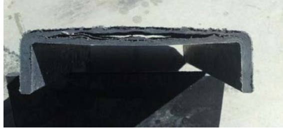
Delamination of a pultruded channel
